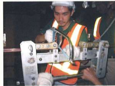
Overhead Catenary System (OCS) maintenance staff on-the-job training on Section Insulator Installation at Depot OCS Training Track.
