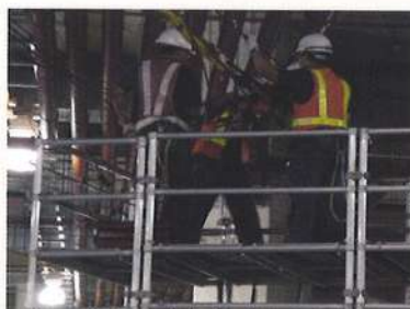
Overhead Catenary System (OCS) dewirement assessment conducted by MTRC HK consultant at Depot Training Track.
