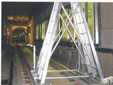
Overhead Catenary System (OCS) high level inspection along tunnel with aid of A-Frame Trolley.
