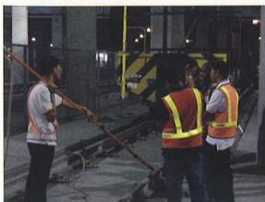
Operations Trainer demonstrating the correct steps to install a Short Circuit Device at Sengkang Depot Training Track.
